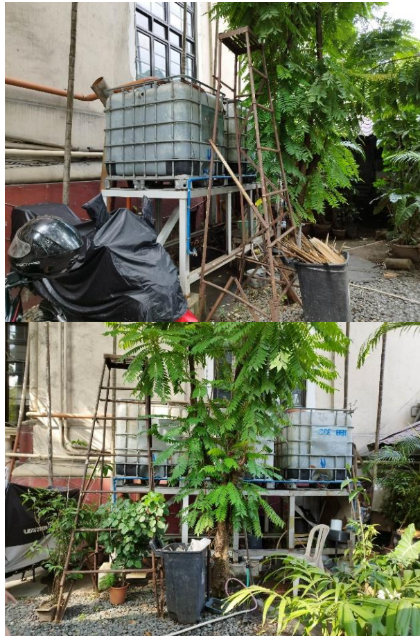
Figure 102 Existing Rainwater Collector Tank located at Rizal Hall, College of Arts and Sciences
